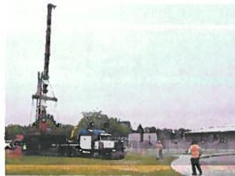
Construction crews install a cell tower next to the Harbour... (Chris Epting)
