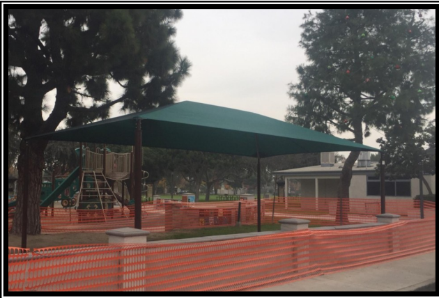
The New Shade Canopy has been installed at the Rush Park Tot Lot.
